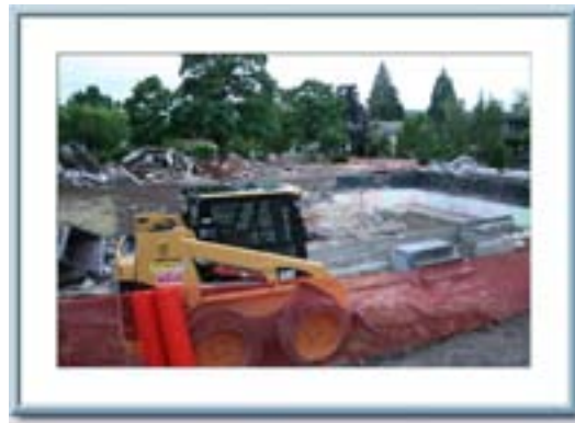
19th and Alder is planned as a 4-story, 96 bedroom building with 17 parking places.
